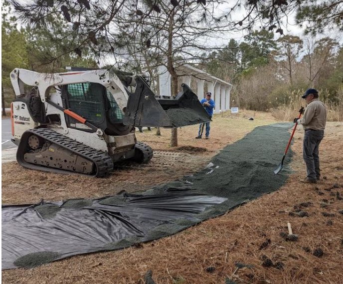
Rebuilding the path around the gardens from the parking lot to the Visitors Center. Lots of help from Chincoteague Fish and Wildlife was much appreciated.
