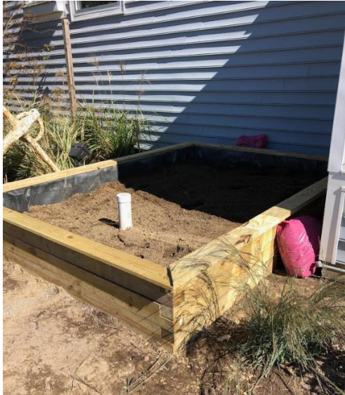
Successful construction/installation of the first rain garden at the Museum of Chincoteague.
