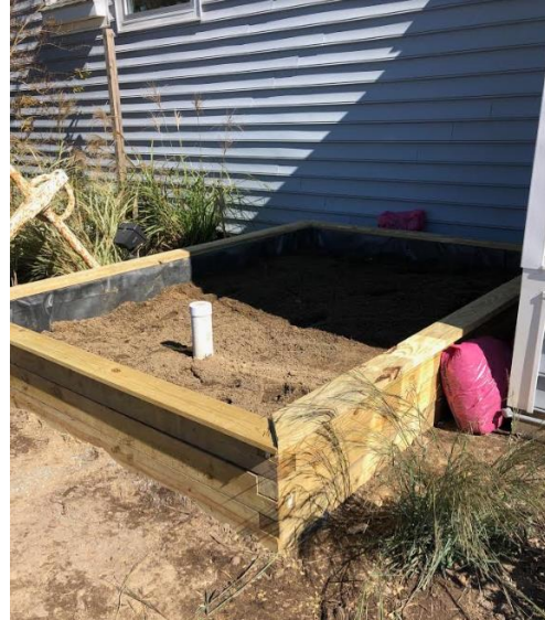
Successful construction/installation of the first rain garden. A 2 nd rain garden is planned for 2020.
